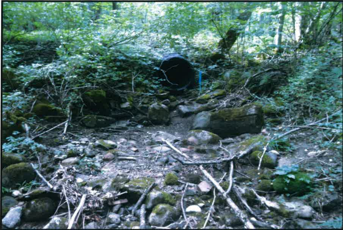
Photograph 1) View of the culvert extending under Collins-Gifford Valley Road. Area 19 extends between the culvert and Woodward Lske.
